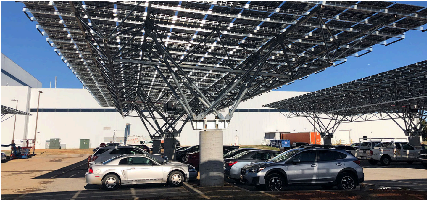
A solar canopy above a parking lot at AVX Corporation in Fountain Inn, South Carolina (photo by Hannah Solar)
